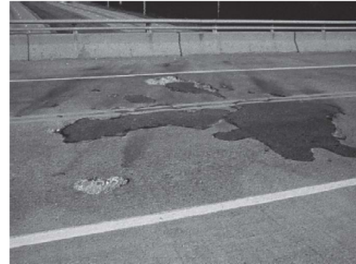
Photo 1 - Spalls and Distressed Patches in Span 2 Deck
