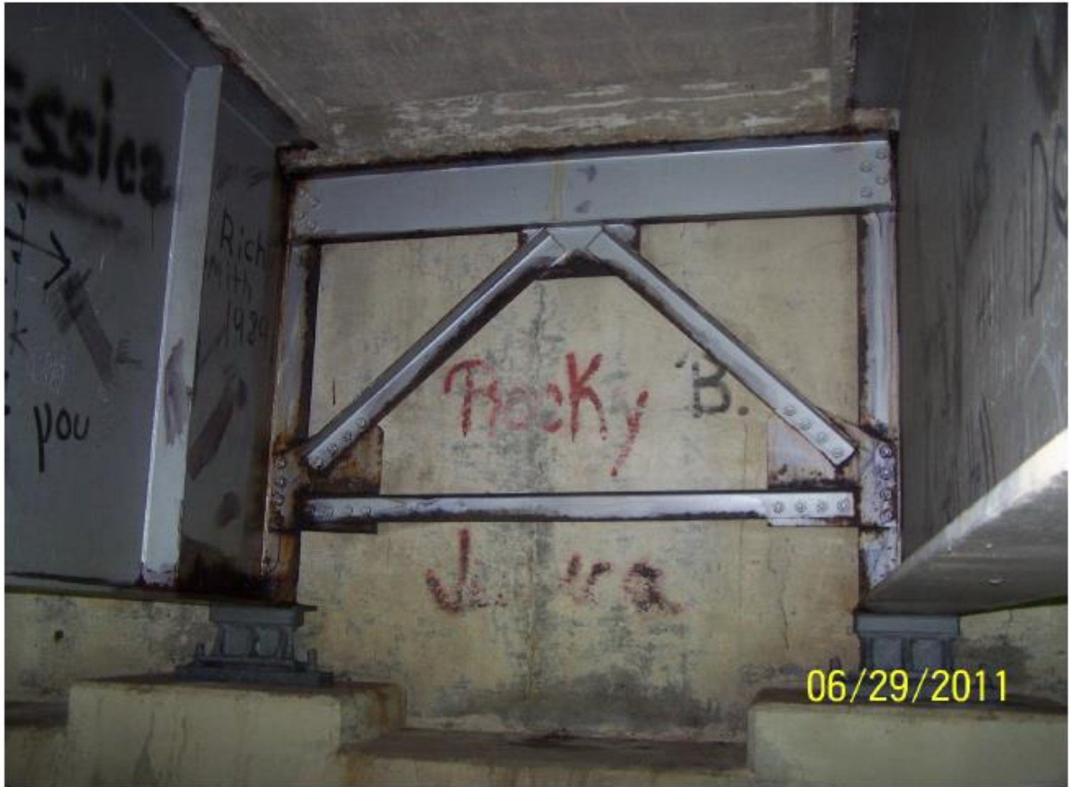
Beam ends and abutment after cleaning and application of black-max and grease (Never-Seez)
