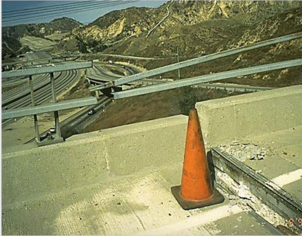
Figure 68: Vertical displacement observed in expansion joint ( NISEE )
