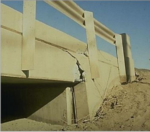
Figure 86: Cracking and rotation of wingwall (NISEE)
