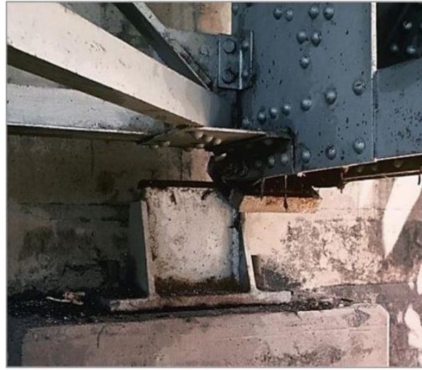
Figure 79: Failure of bearing, complete lateral displacement ( NISEE )
