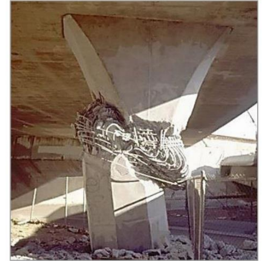
Figure 93: Failure of column (NISEE)
