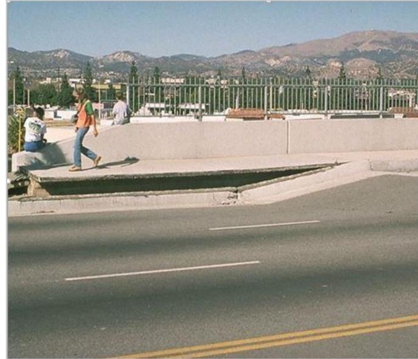
Figure 63: Settlement of the approach slab ( NYSDOT )
