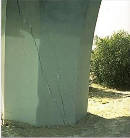
Figure 94: Shear cracks in column ( NISEE )
