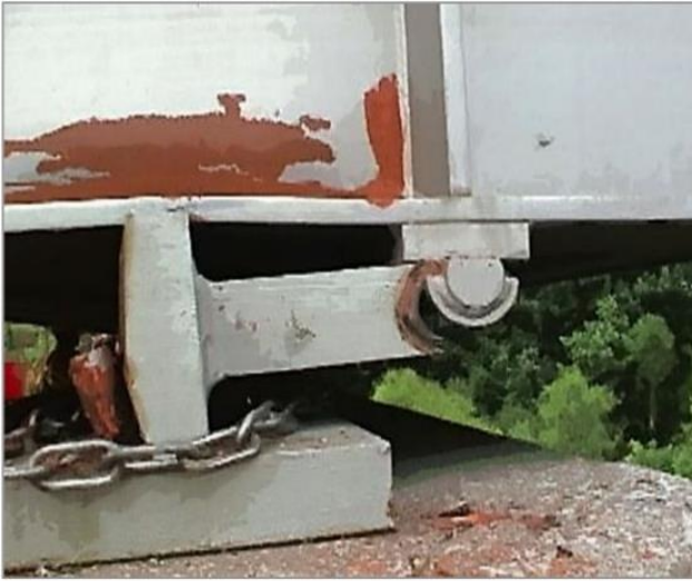
Figure 78: Rocker bearing failure ( NISEE )
