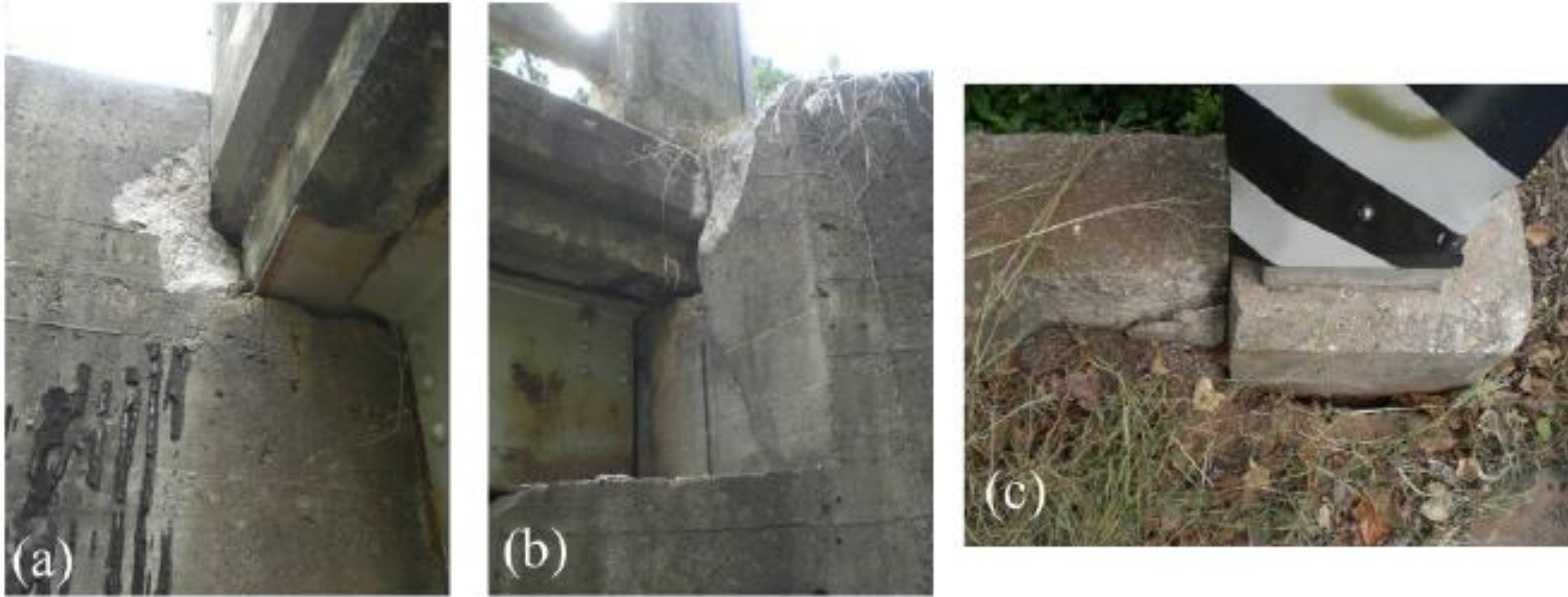
Figure 14: Observations of damage at the West Abutment of Belford Bridge (Latitude/Longitude: (36.505°, -96.8493°)): a,b) concrete spalling of abutment; c) approx. 4 cm wide gap between backfill soil and abutment
