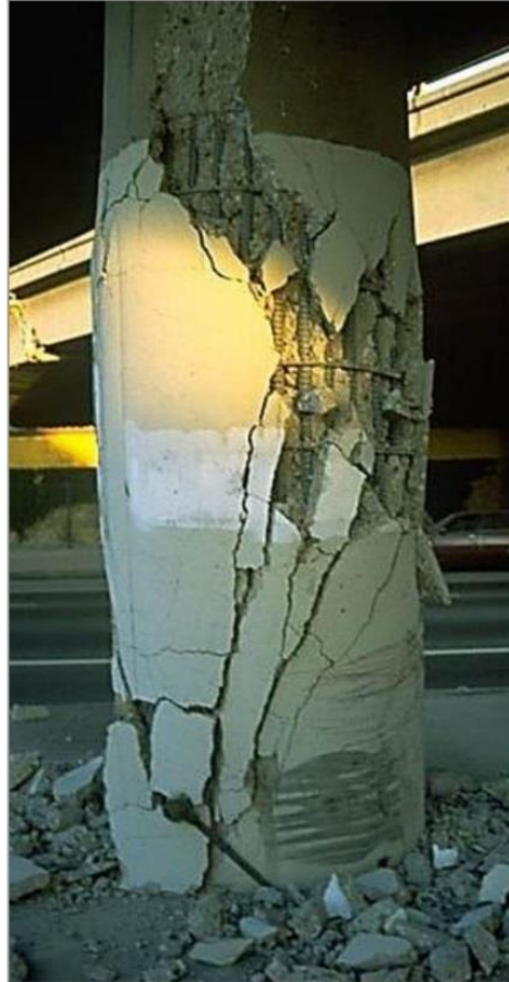
Figure 96: Confinement failure in single column ( NISEE )
