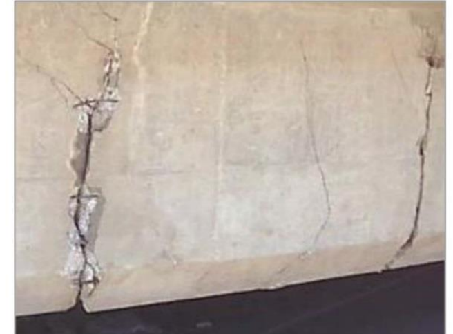
Figure 74: Cracking in web of concrete beams ( NYSDOT )
