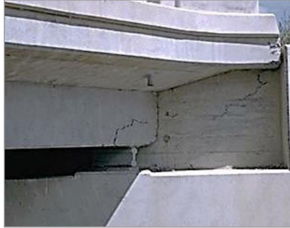
Figure 77: Superstructure spalled at bearing location ( NISEE )
