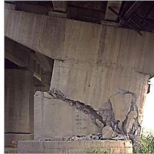
Figure 92: Full collapse of pier (NISEE)
