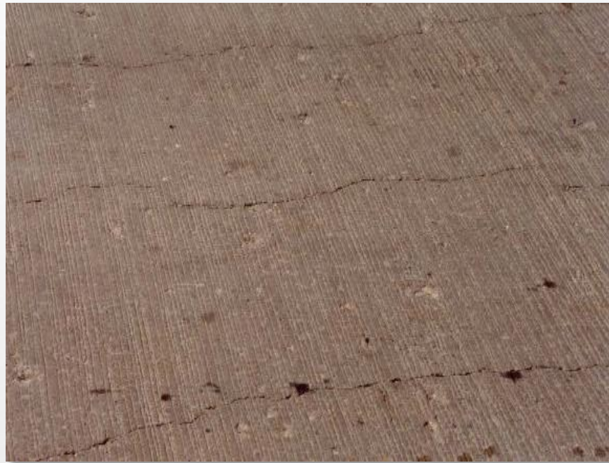
Cracking (shrinkage, ASR, loading)
