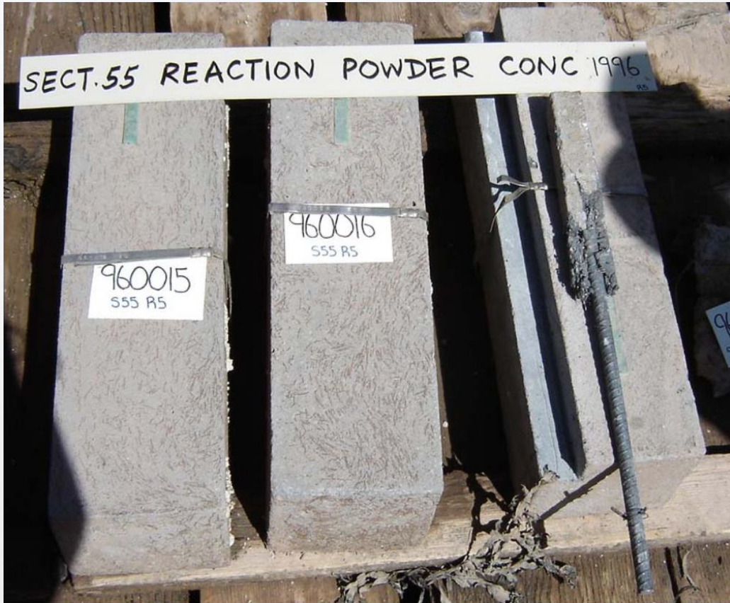
In 2006 – Rebar at 10-mm (3/8-inch) cover removed from one of the 10-year-old beams
