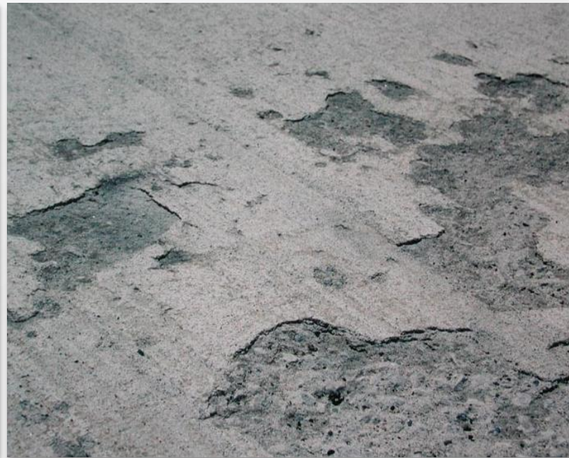
Spalling (freeze/thaw, carbonation, corrosion)
