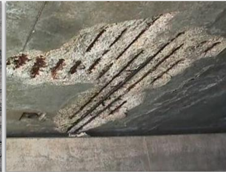
Corrosion (chloride/acid penetration)
