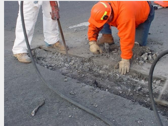
Clean out the rubble. The crew is taking care to not hammer the rebar.
