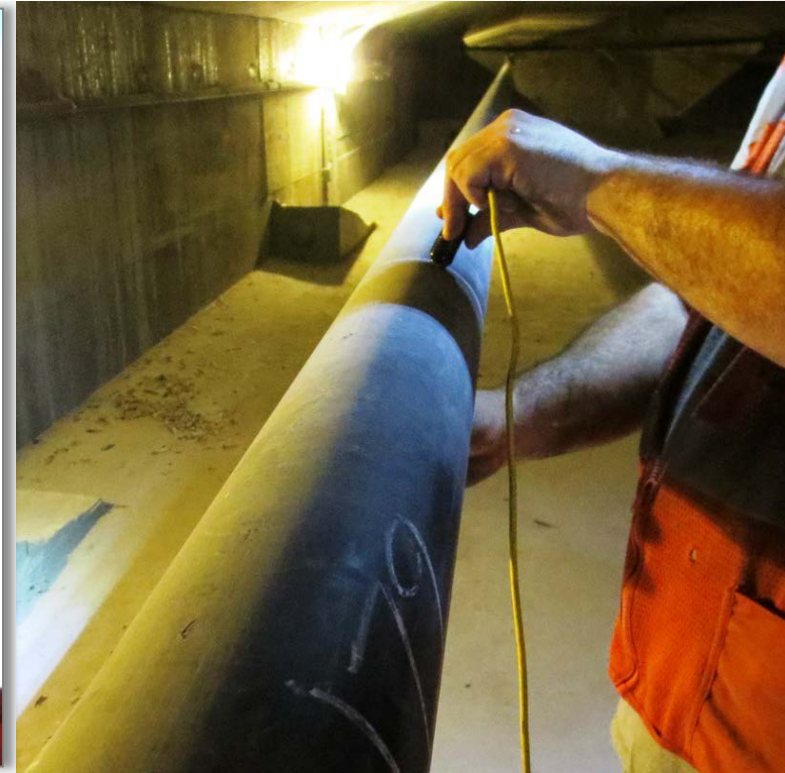
External PT Ducts
