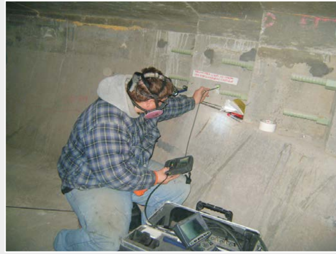
Document Internal PT Duct Conditions
