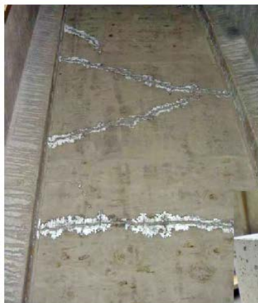
Full-Depth Shrinkage Cracking on Prestressed Girder Bridge
