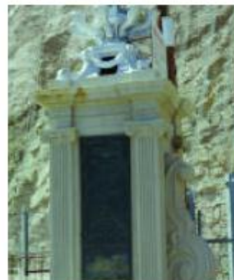
Top: Pylon before rehabilitation in 1995. Center and bottom: Pylon in September 2004. There is minor rust staining from the fixture above. Completely intact as completed in 1995 with some small rust stain bleeding from above.
