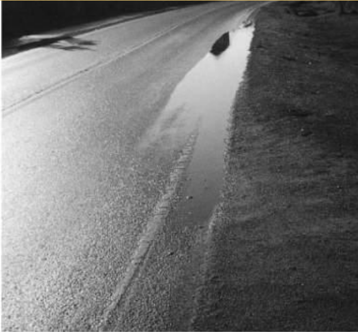
Water ponding at the edge of roadway.
