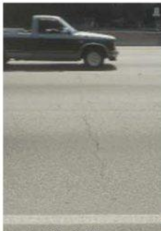
Low to Mod. Transverse Cracking
