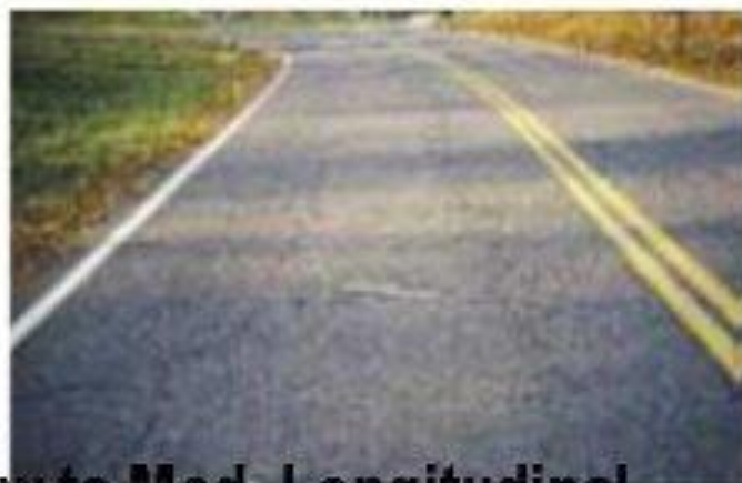
Low to Mod. Longitudinal Cracking
