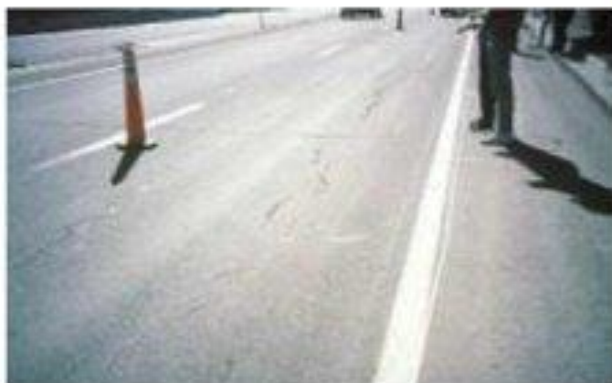
Low Severity Wheelpath
