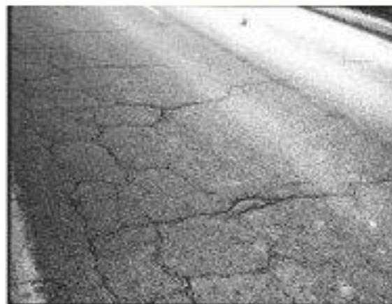
High severity block cracking
